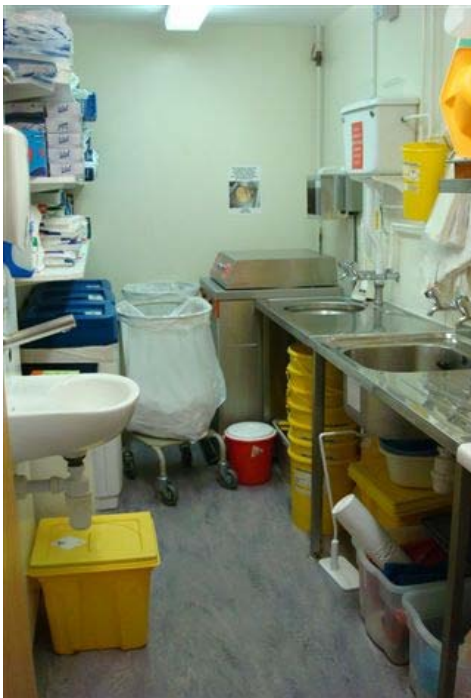
Kingfisher Ward sluice
